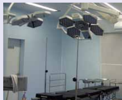
Guided Airflow Ultraclean Operating Room, Johnson Trivitron OT solutions, India.
